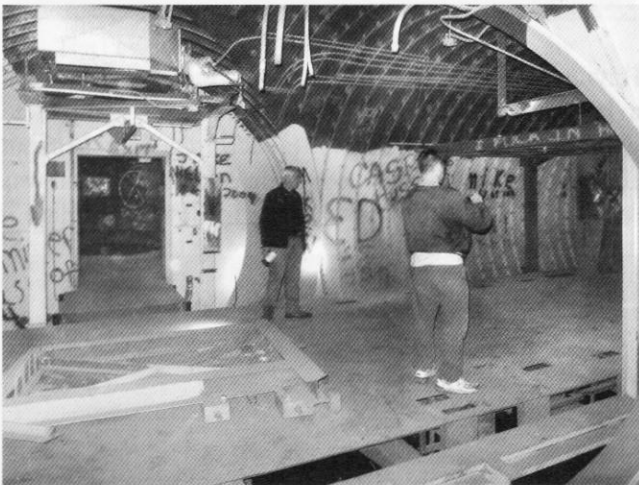
The antenna tunnel junction. One of the antenna silos is visible on the left
